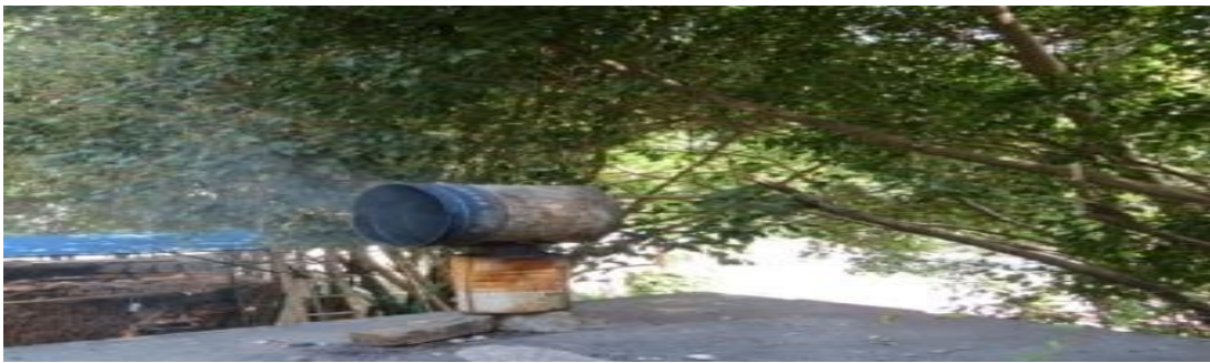
Fig. 2 The long chimney connected to cooking stove crossing the flat roof with trees growing toward it.
